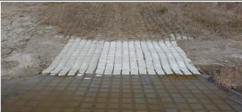
Photograph 2 (South perimeter berm downstream slope and south ditch) Downchute channel and recently constructed hydraulic jump basin in good condition. (IMG_DSCF1747.JPG)
