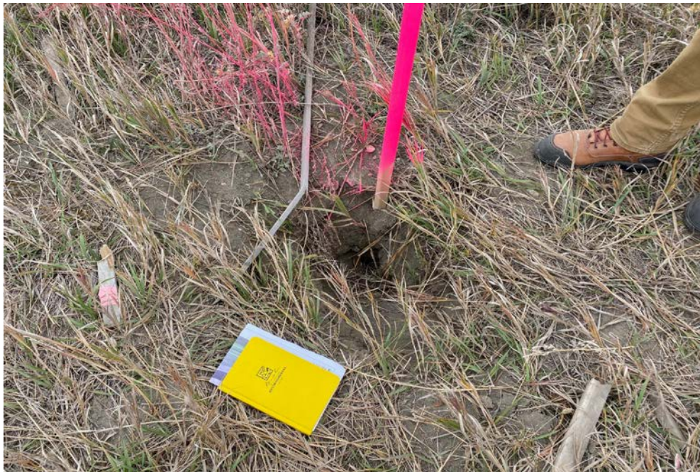
Photograph 20 (South perimeter berm downstream slope) Animal burrow. (IMG_AD11P.JPG)
