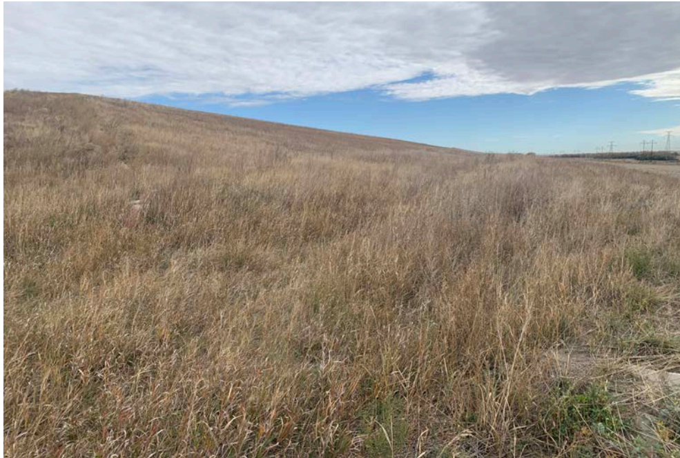
Photograph 15 (South CCR downstream slope (final cover)) Well-vegetated final cover terrace channel. (IMG_4638.JPG)
