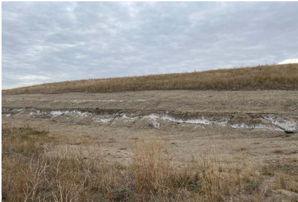
Photograph 17 (North CCR downstream slope (no cover/temporary cover)) Temporary cover and contact water contaminant channel. (IMG_AD14P.JPG)
