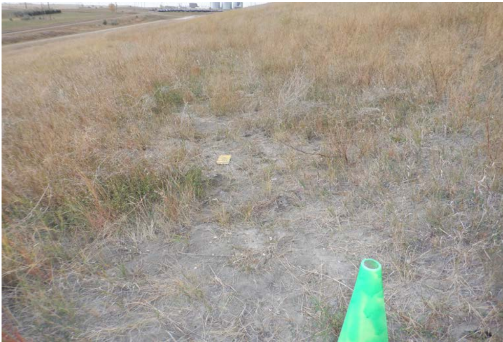
Photograph 1 (South CCR Downstream Slope (covered)) Animal burrows and sparse vegetation on downstream slope. (IMG_DSCF1743.JPG)
