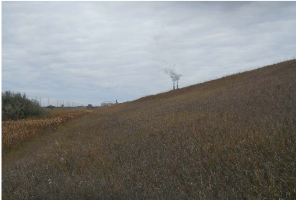
Photograph 21 (South perimeter berm downstream slope) Well-vegetated (grass) perimeter berm downstream slope. (IMG_AD16.JPG)
