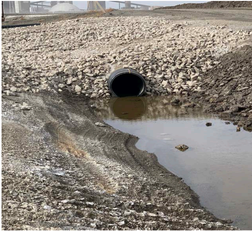
Photograph 9 (North CCR downstream slope) Perimeter contact water channel and culvert to Upstream Raise 91. (IMG_BP15.JPG)
