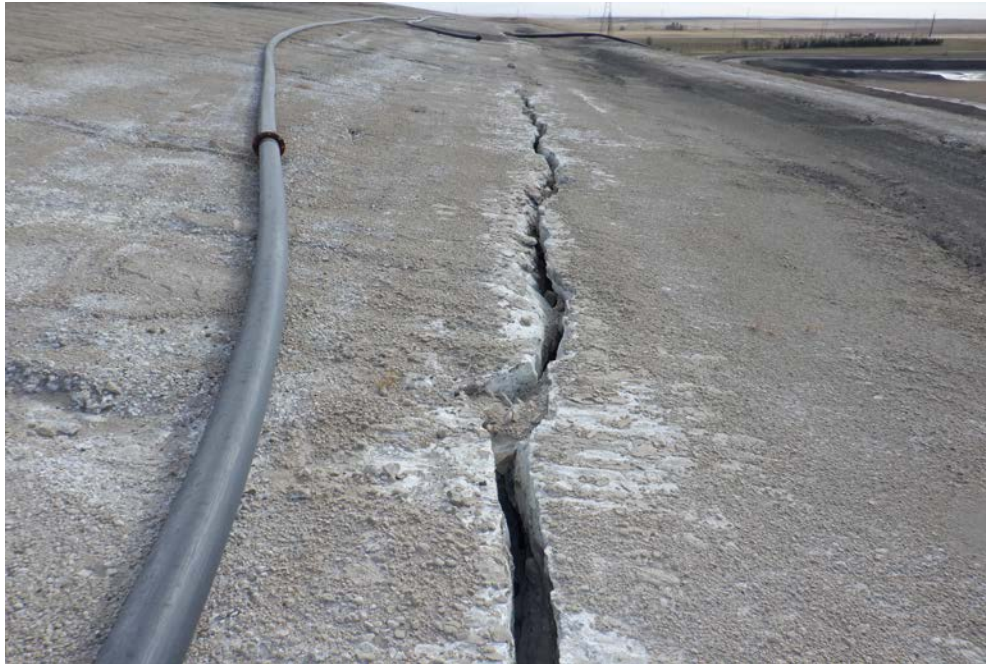
Photograph 5 (West CCR downstream slope (no cover)) Approximately 6-inch wide crack in fly ash within the bench at elevation 1974 feet. (IMG_DSCF1757.JPG)
