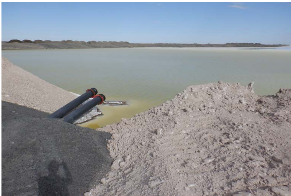
Photograph 6 (East CCR upstream slope (no cover)) Gravity drain piping inlet to Upstream Raise 91. (IMG_DSCF1767.JPG)
