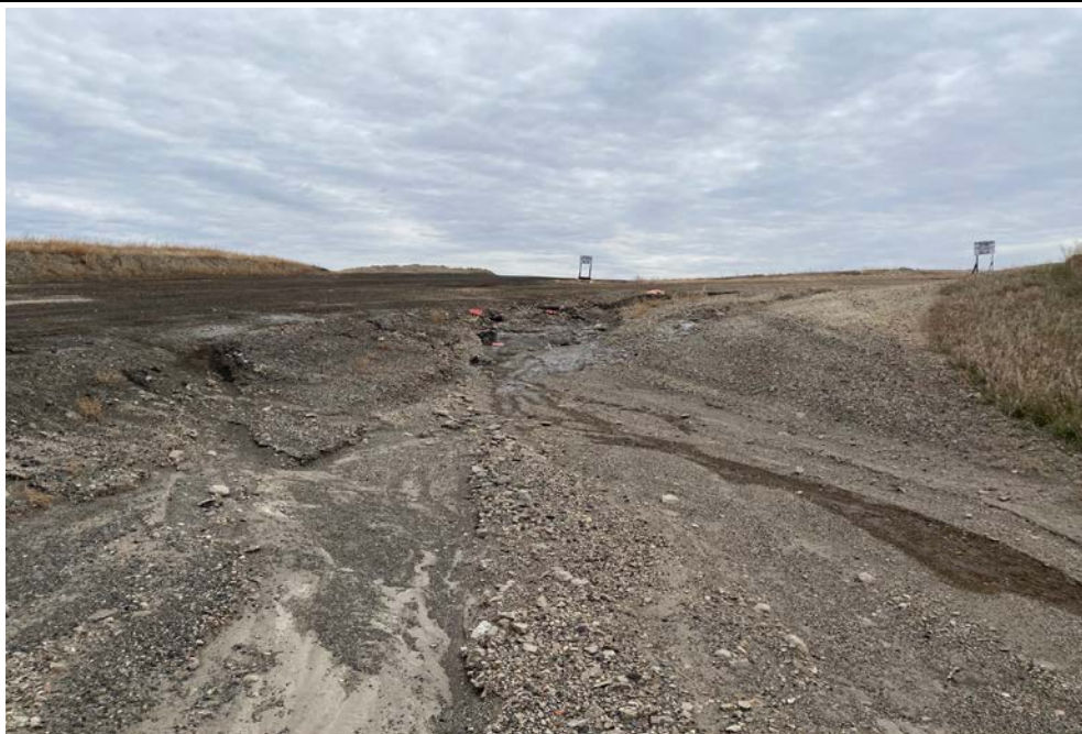
Photograph 18 (East CCR upstream slope (road)) Erosion on the corner of the main east/west haul route to the southeast corner of Upstream Raise 92. (IMG_AD15P.JPG)
