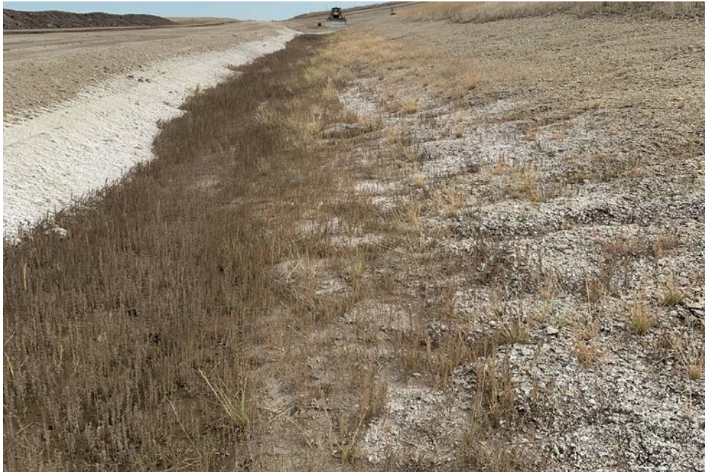
Photograph 14 (North CCR downstream slope (no cover)) Contact water channel with sparse vegetation. (IMG_DP14.JPG)
