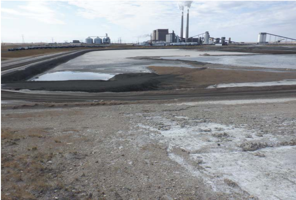
Photograph 7 (West CCR downstream slope) Minor erosion of fly ash in southwest corner between elevations 1950 feet and 1974 feet. (IMG_DSCF1762.JPG)
