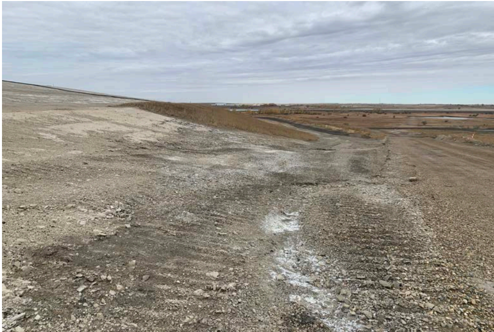
Photograph 13 (East CCR downstream slope (no cover)) Minor fly ash erosion on the east slope above the haul road. (IMG_DP1.JPG)
