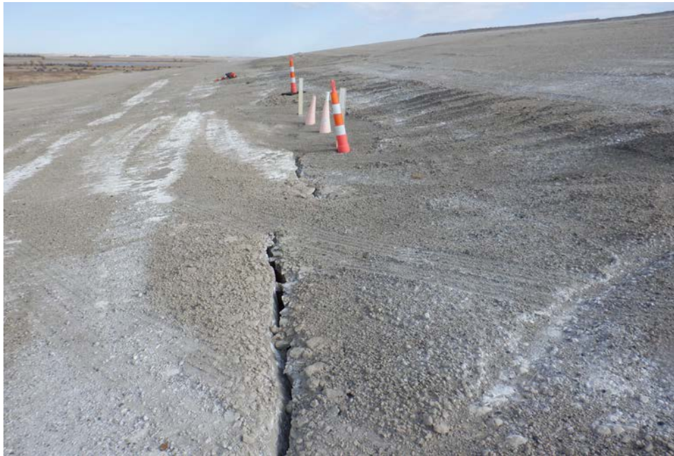
Photograph 10 (North CCR downstream slope (no cover)) Cracking and erosion of fly ash around piezometers. (IMG_DSCF1774.JPG)
