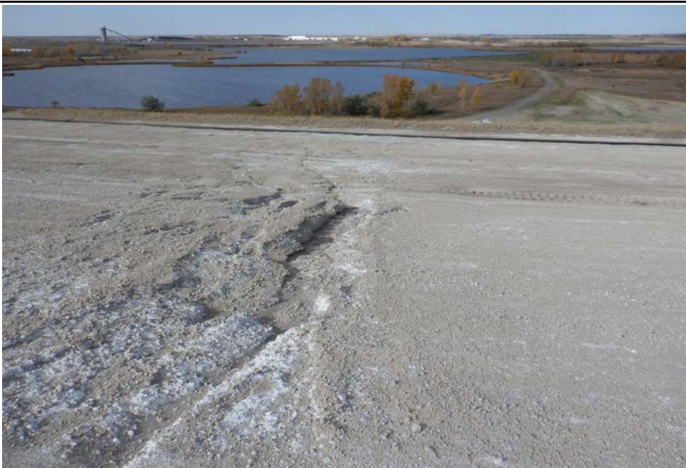
Photograph 8 (North CCR downstream slope) Erosion of fly ash below elevation 1998 feet. (IMG_DSCF1771.JPG)
