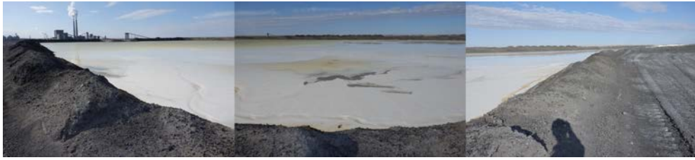
Photograph 11 (South CCR upstream slope ) Panoramic of Upstream Raise 92 CCR upstream slope and FGD pool. (IMG_DSCF1787-1789.JPG)
